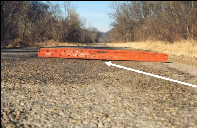
\frac{3}{4} inch (19 mm) rut in "outer wheel path"
