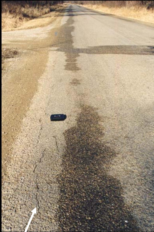
Cracks along shoulder
